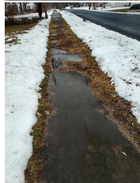
Examples of cracked, overgrown, and flooded sidewalks
