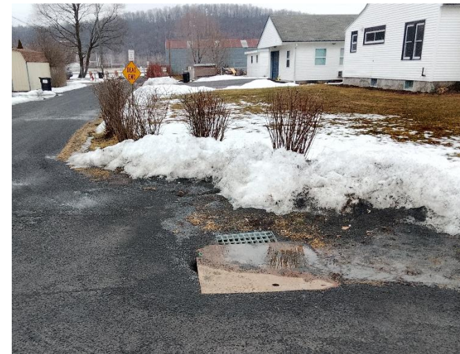
A large hole has formed where stormwater pools around a catch basin at the corner of Prospect Place and Speedway
