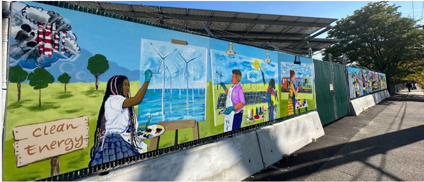
NineDot community storage installation sited across the street from a school in the Bronx
