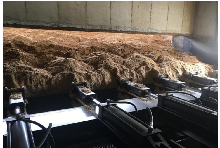
Sawdust utilized for boiler fuel in Wagner facilities.
