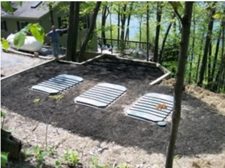
Photograph: Peat moss modules installed at a lakeshore residence. These modules receive effluent from the septic tank, promote enhanced pathogen removal, and discharge effluent to the absorption field.
